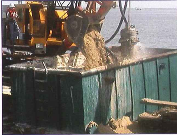
Pump in a box.
