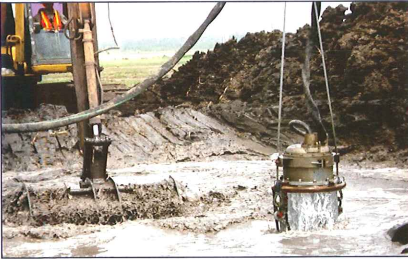
Pump in a pit - Restoring wetlands
