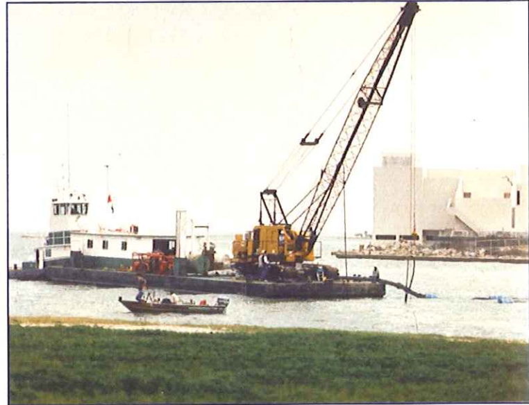
Pipeline uncovered in the Corpus Christi Ship Channel
